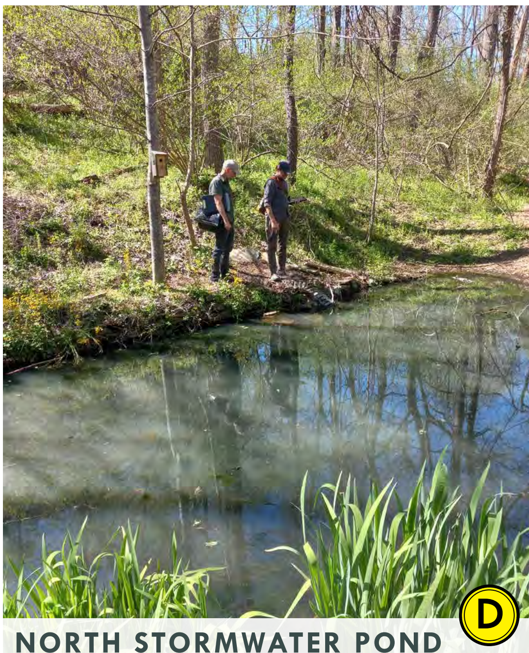
NORTH STORMWATER POND
